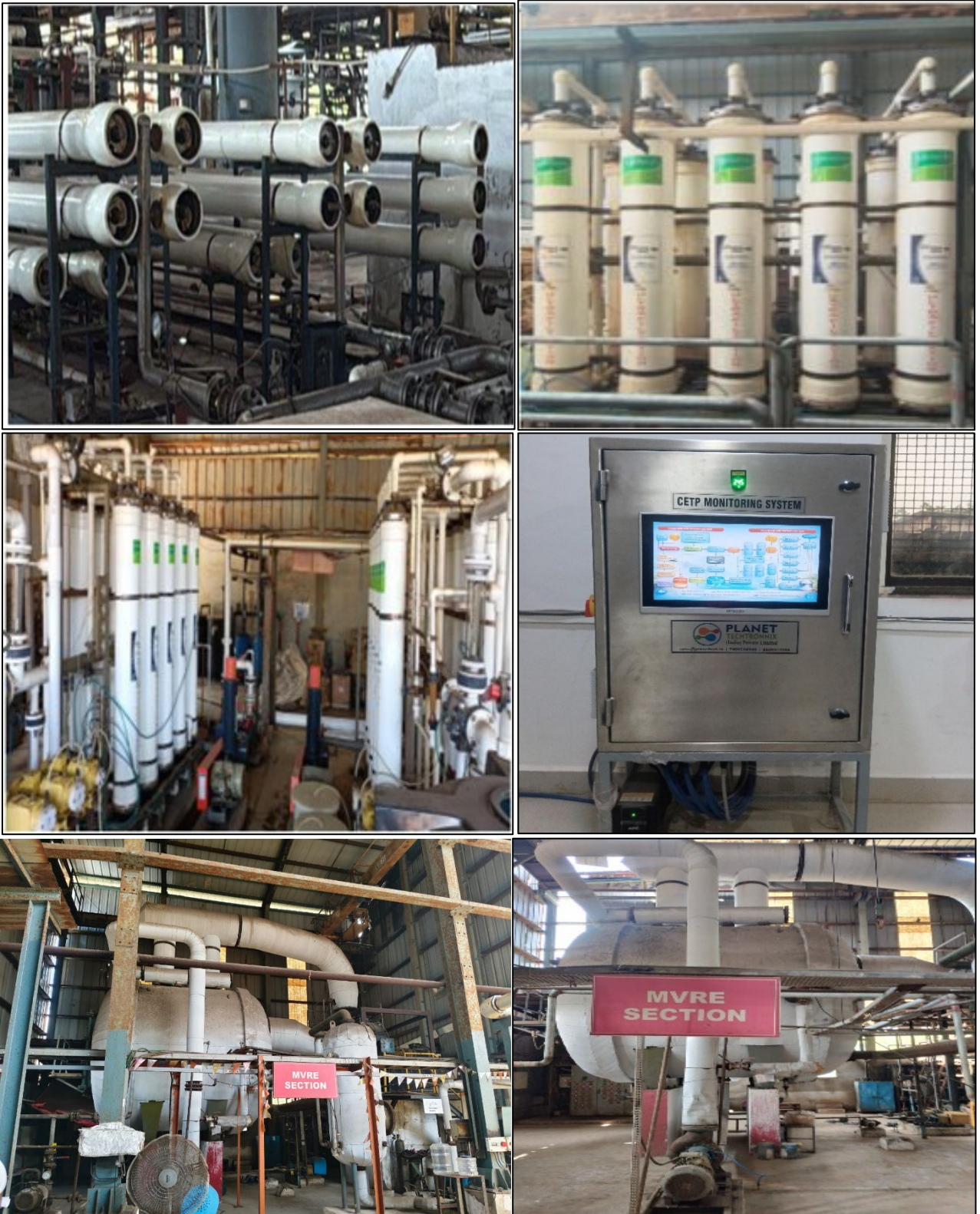
Effluent Treatment Plant with UF, RO and MVRE
